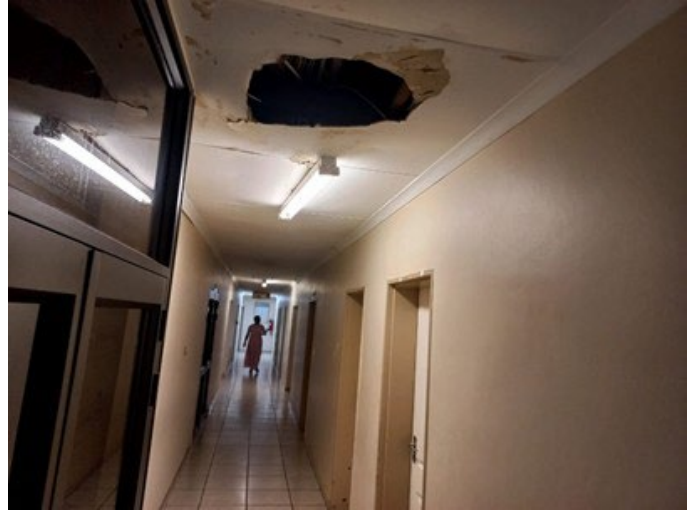
Figure 4: Dilapidated municipal offices, Thembesile Hani Local Municipality. Source: Photograph taken by Taki Sithagu, 2023.
